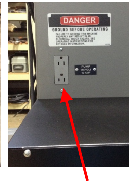
120VAC receptacle for pump
